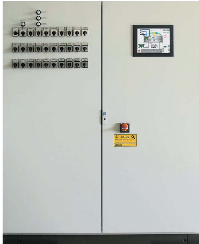
The heart and brain of your biogas plant: The switch cabinet with central control via display
