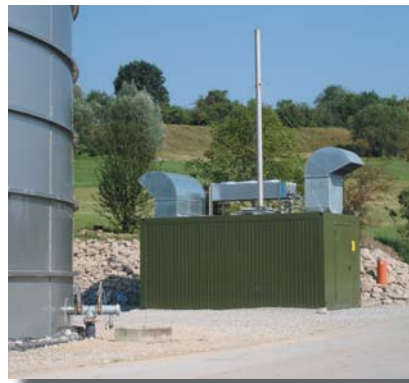
Thermal power station in modular design
